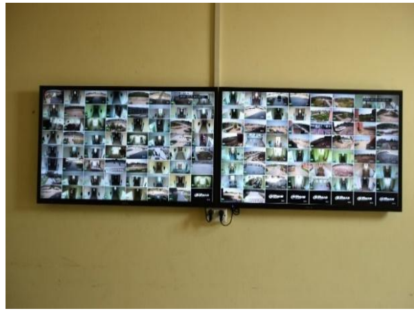
Video Surveillance Room
