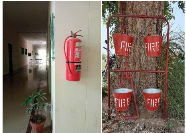
Installed: Fire Extinguishers and Fire Buckets
